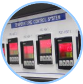
Board's Heating System
